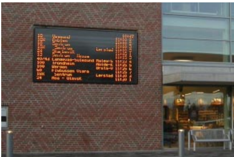
The new LED-display at Moa Bus station in Ålesund is connected to PATServer information system.
